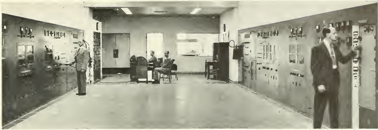
TRANSMITTER PANELS LINE BOTH SIDES OF THE CONTROL ROOM OF THE SHORT-WAVE PLANT AT DIXON, CALIFORNIA.
